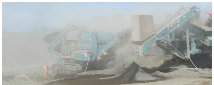
Prior to the installation of Polo BDS, dust emissions around the mobile plant made visibility extremely difficult.
